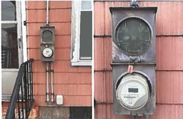
Outside Electrical Meters - (2)
