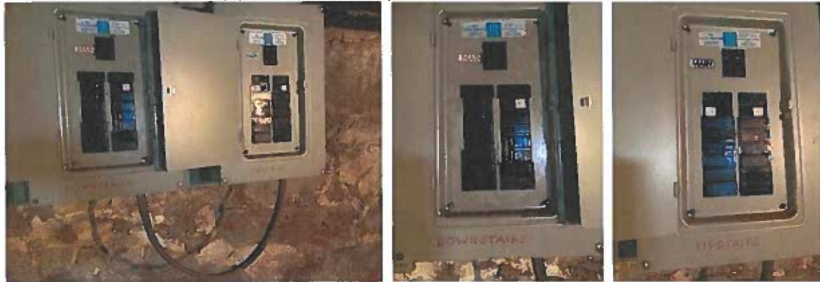
Inside Electrical Panels - (2) Downstairs & Upstairs
