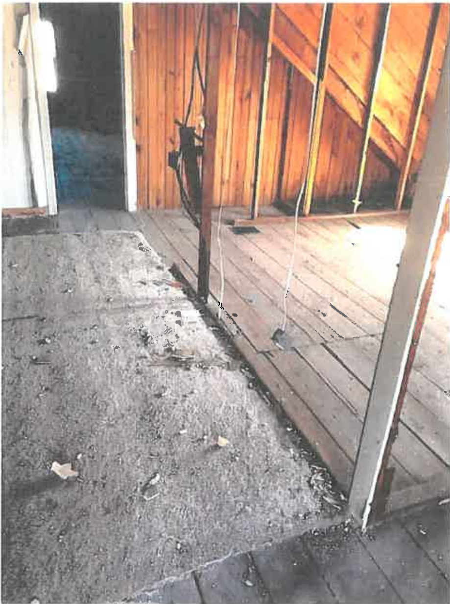
EXHIBIT E - 3rd Floor Showing Dangling Electrical Boxes and Original Flooring
